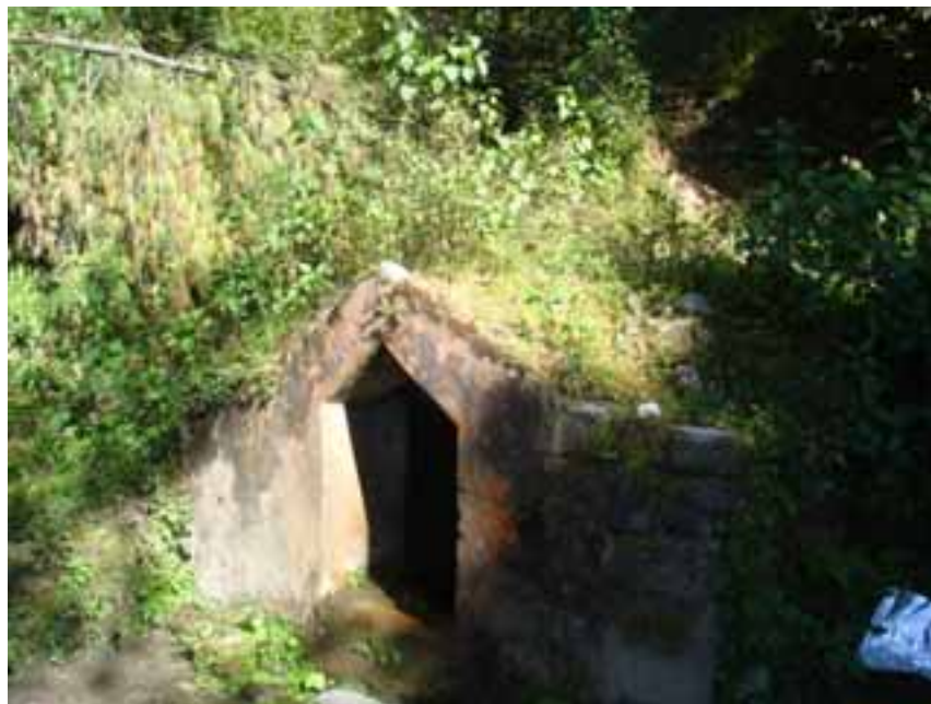
Figure 3: Storage structure to collect spring water in Nagarkot hills close to Kathmandu valley area (from field visit during sensitization trip)
